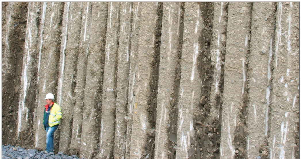
Oasys software was used to design buttressed piles to support a three storey basement in Ireland
